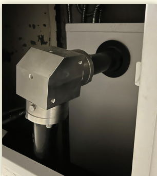
2" DoubleTrac fuel oil fill from Simplex Fill Station
