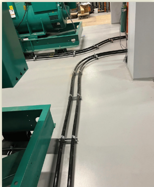
1" DoubleTrac ® fuel oil supply and 1" DoubleTrac fuel oil return piping from Day Tanks to Generators.
