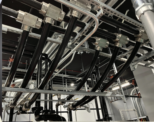
2" DoubleTrac ® piping and 2" DoubleTrac ® tees over generator pads
